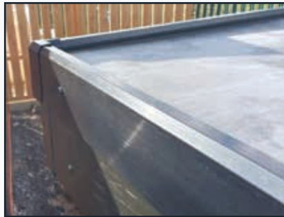
EPDM maintenance free synthetic one piece rubber membrane covering the roof
